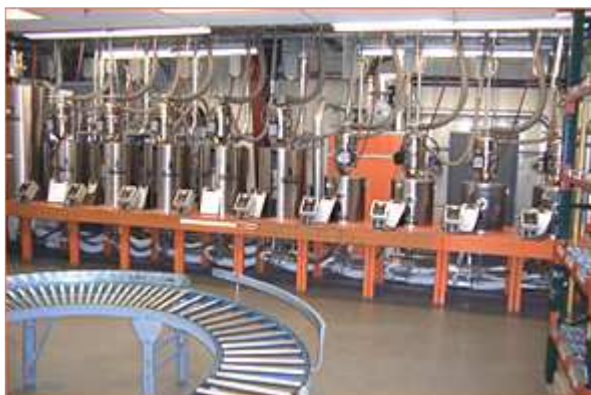
A row of standardized Motan dryers at GW's plant in Bethel, Vt.
